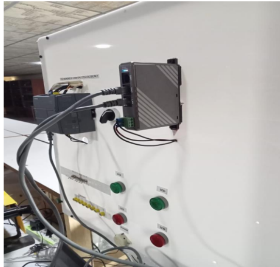
Figure 3-8 IOT Gateway with temp control system.
